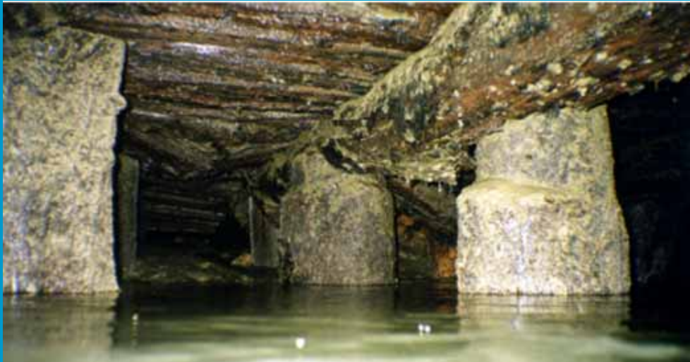
Fungal attack of beech piles and caps, Rouen Harbor
